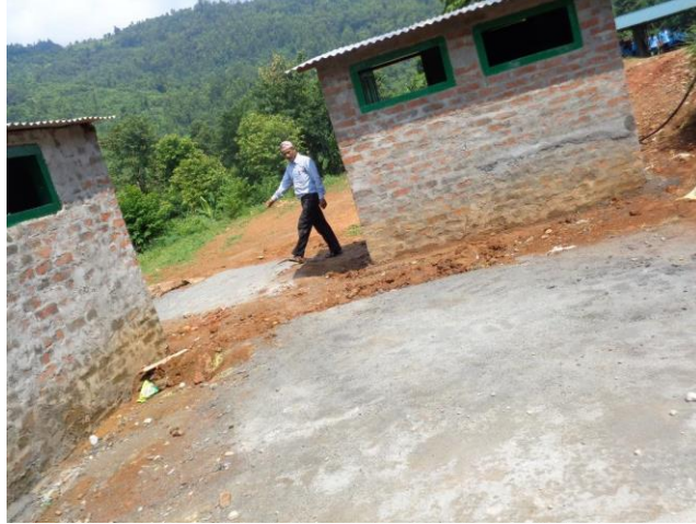
Fig: Toilets with water supply facility
