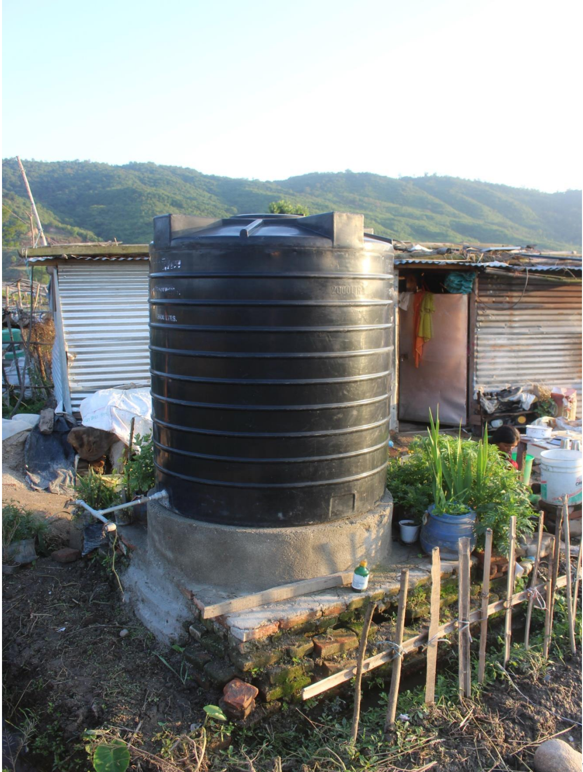
Reserve tank to supply drinking water to the local villagers
