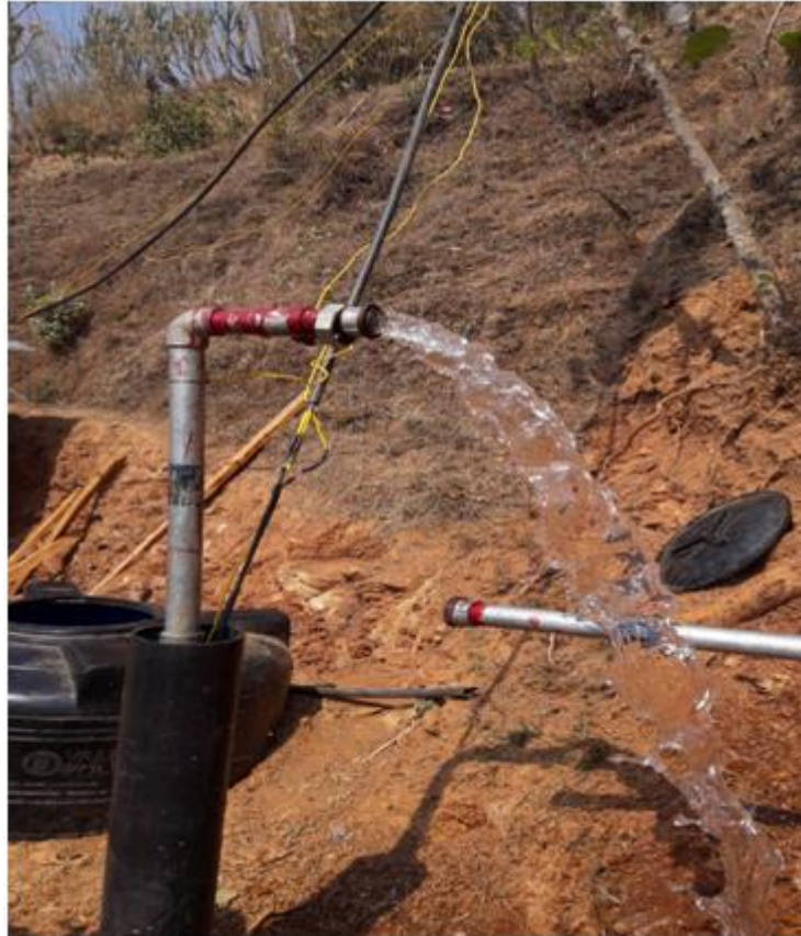
Water flowing through a main pipe at Thansing
