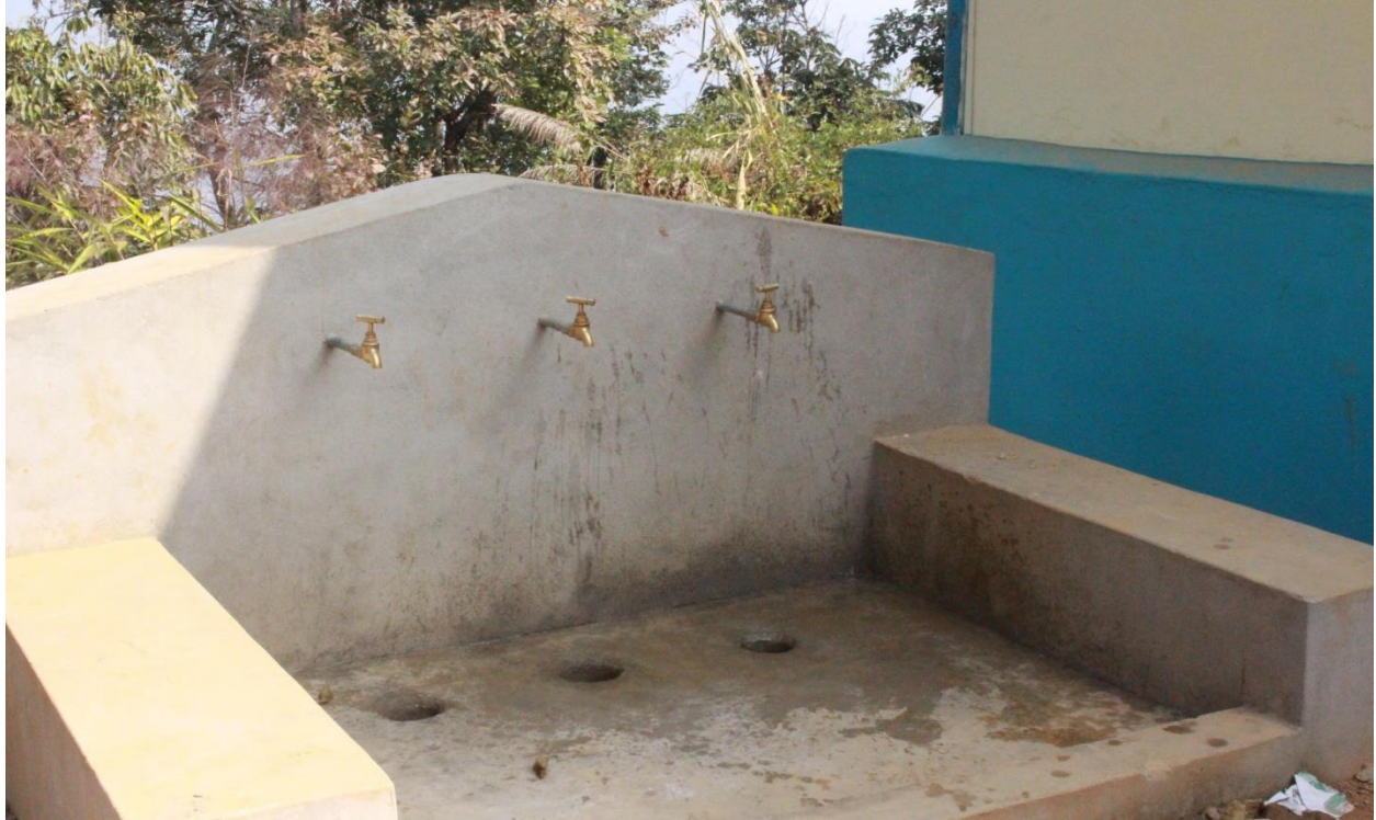
Drinking water supply at Om Ram
